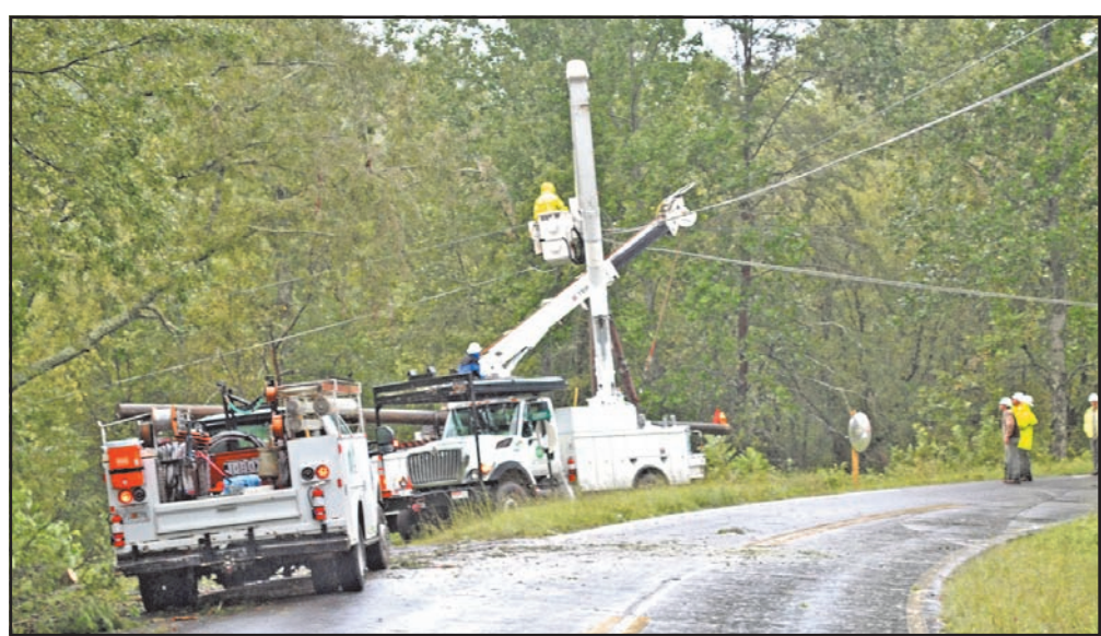
Blue Ridge Mountain EMC workers fixing a broken power pole on Fodder Creek Road in the aftermath of Hurricane Irma. Photo/Lowell Nicholson
